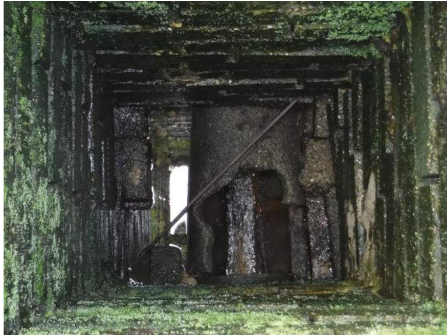
Image 5: Concrete pipe conveys flows through this CB
