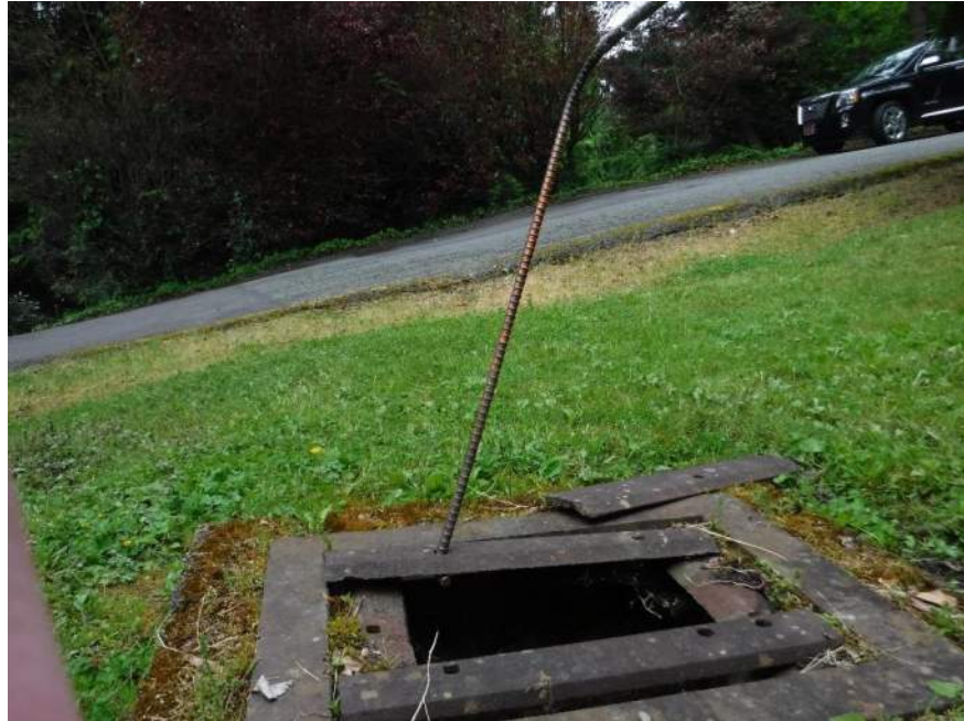
Image 3: Flows enter this CB located just northwest of W Mercer Way
